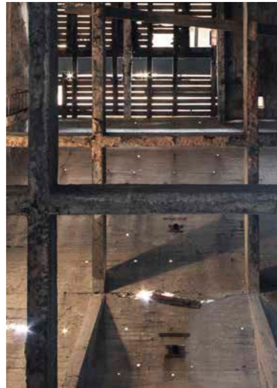
The star-like piercings in the concrete skin, to be filled with glass pegs
