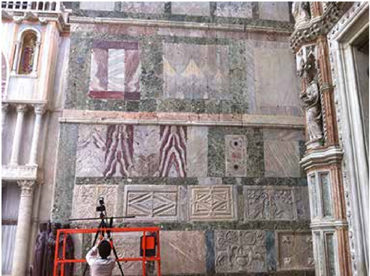
1 View of the south exterior wall of the Treasury of San Marco, Venice
