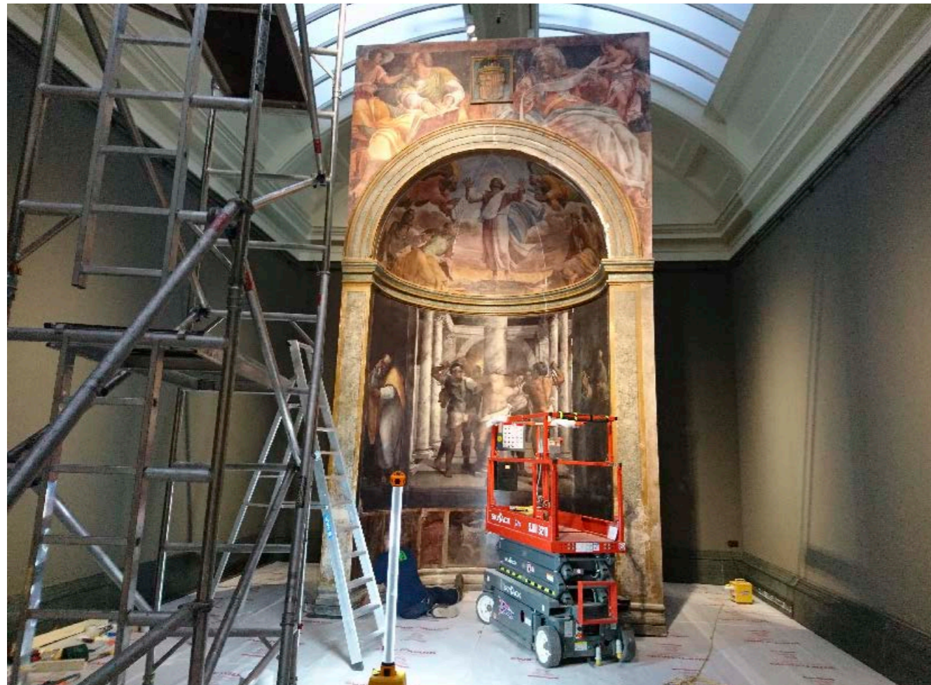
Installing the replica of the Borgherini Chapel, from the convent of San Pietro in Montorio in Rome, inside the National Gallery, 2017
