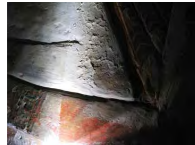
Detail of a restoration carried out in 1999 showing the addition of white paint and the application of an acrylic consolidant. In raking light it is clear that it is now cracking and peeling from the wall.
