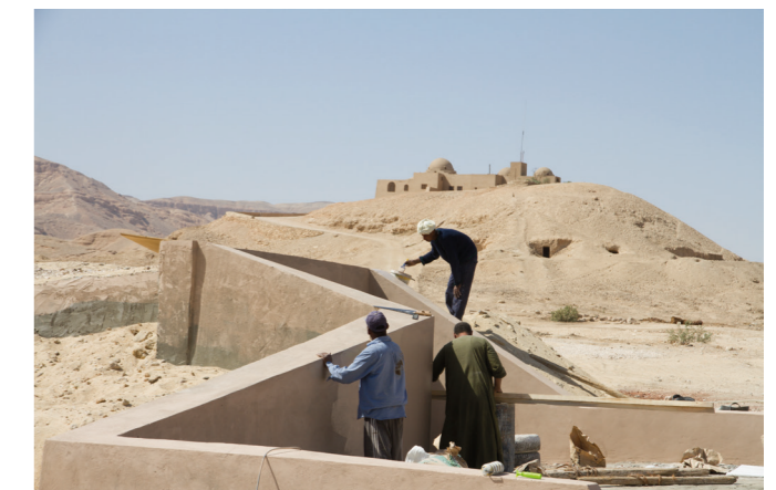
The exterior of the facsimile of Tutankhamun's tomb being worked on with Hassan Fathy's vernacular architecture in the background. Photo: Factum Arte
